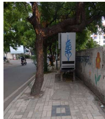
Figure 10- Electric box obstructing walking space on Footpath
